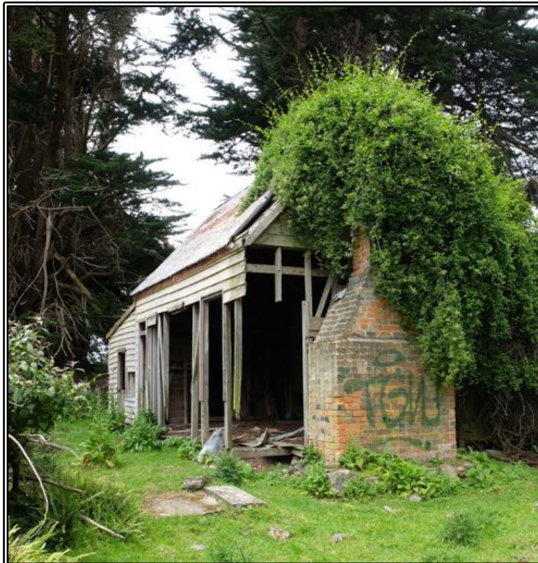
Figure 204 The eastern end of Stewart's cottage, showing the large brick chimney and perilous state of the front framing.
