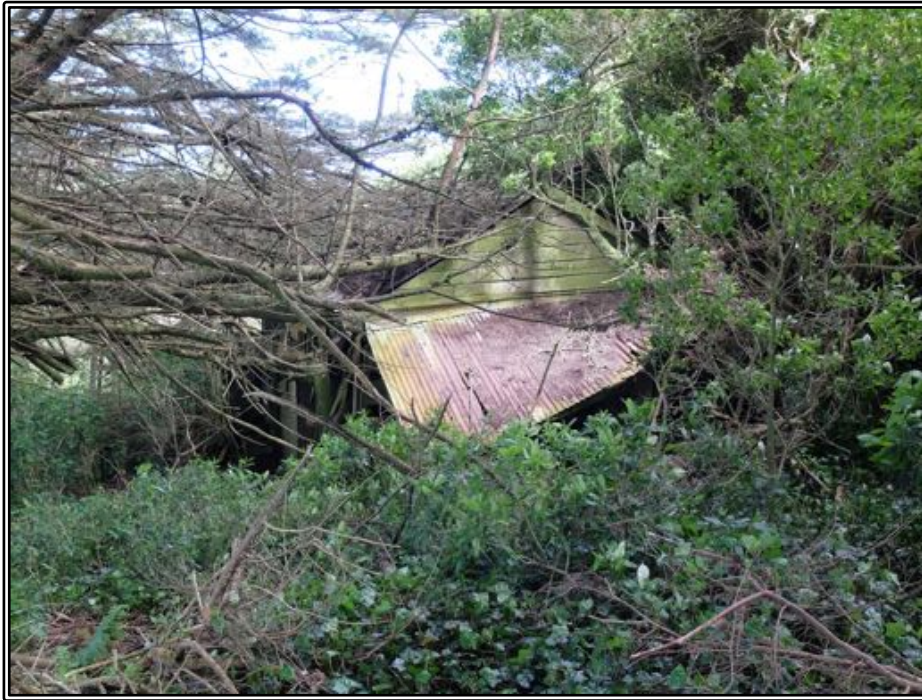
Figure 34 The north end of Riddell's farm building. The building collapse, aided by descending macrocarpa branches, is apparent.
