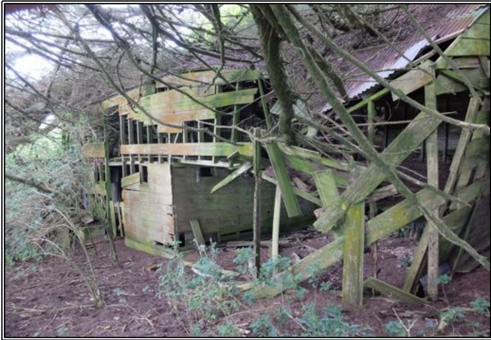
Figure 169 The front (east) wall of Riddell's farm building in 2020, showing the partial collapse of the structure.
