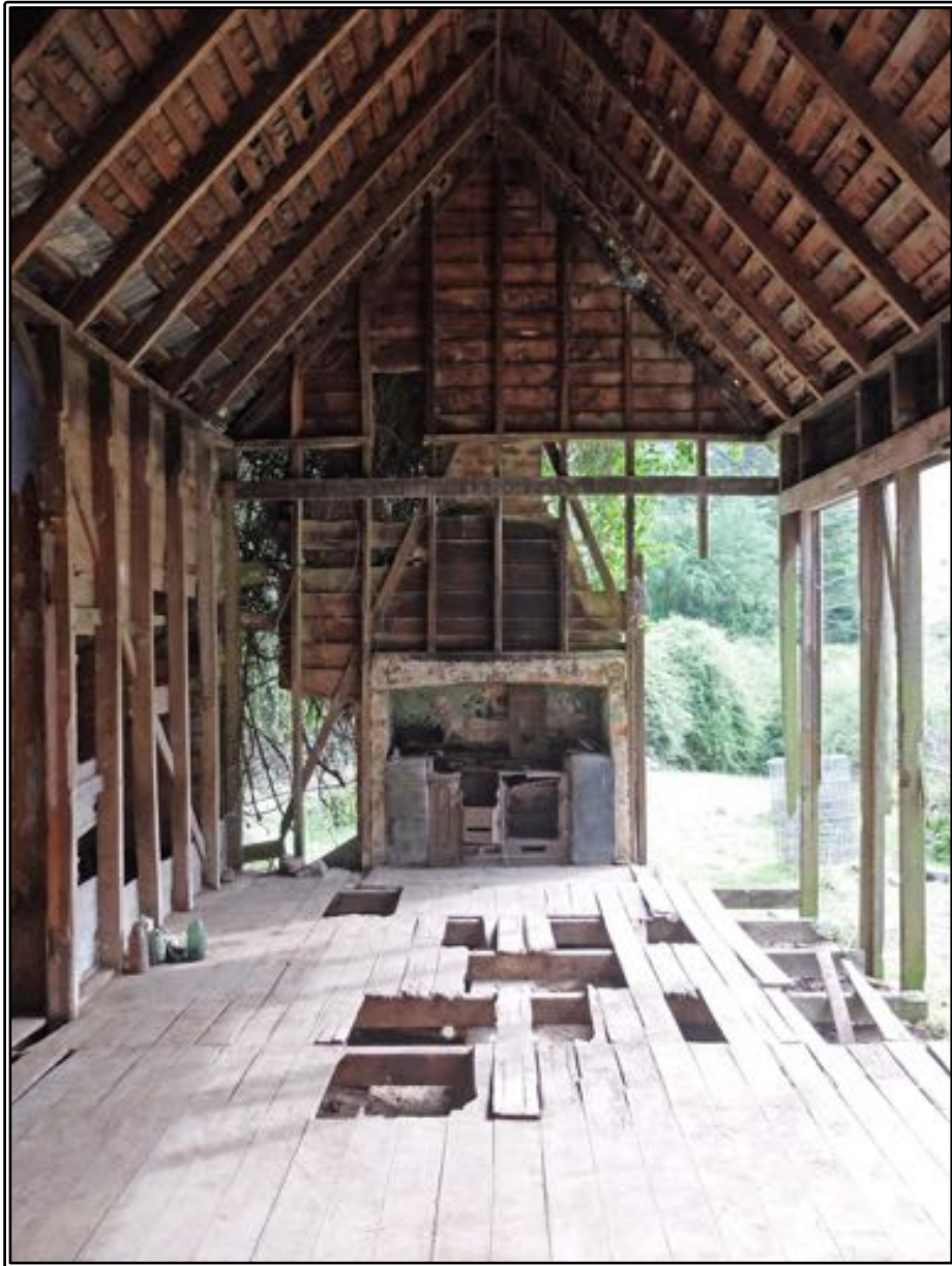
Figure 209 Inside the original section of Stewart's house after it was cleared of sheep droppings and debris, looking towards the west end with the chimney and Shacklock coal range.
