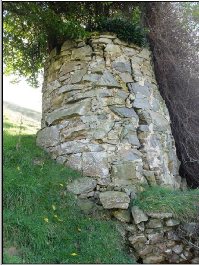
Figure 213 The charging bowl of the limekiln. Note the crack running the full height of the structure.
