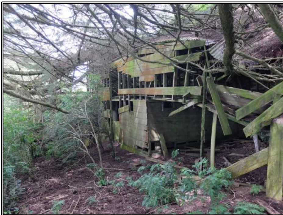
Figure 35 The front of Riddell's barn/byre/stables building. The centre section of the building is still standing, but the far end (south, the byre section) has collapsed after a tree fell through it.
