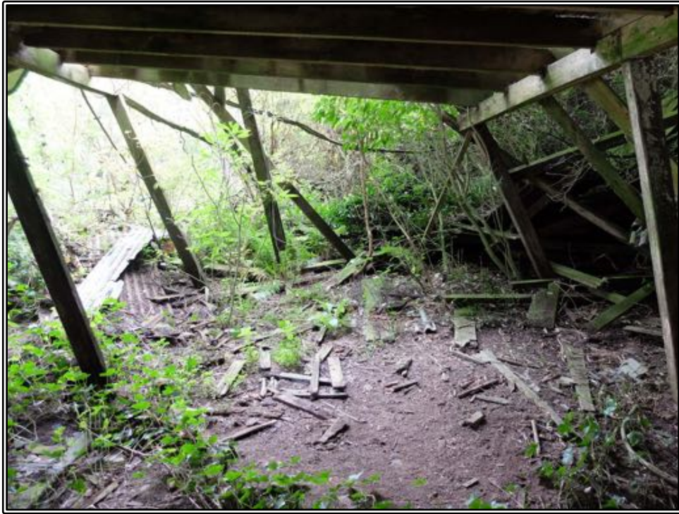
Figure 179 The cow byre, looking south into the collapsed portion of the building.
