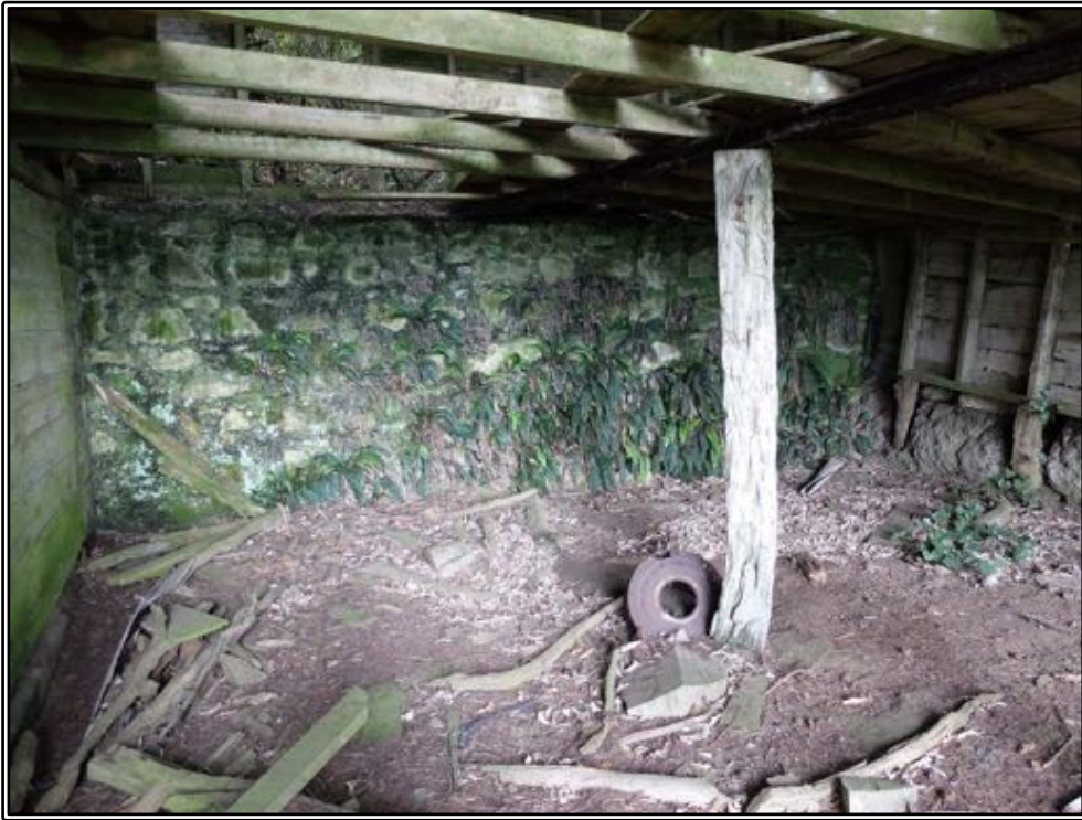
Figure 173 Inside the northern ground floor room of Riddell's farm building, with the stone retaining wall at the rear.
