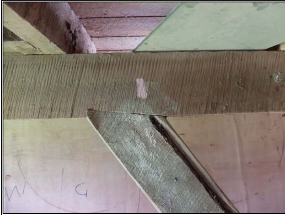
Figure 190 Pit sawing marks on timber framing (floor joist and post brace) in Roger's byre.
