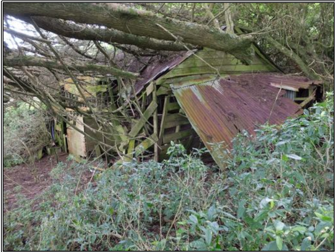
Figure 168 The north end of Riddell's farm building in 2020, showing the partial collapse and damage from macrocarpa limbs.
