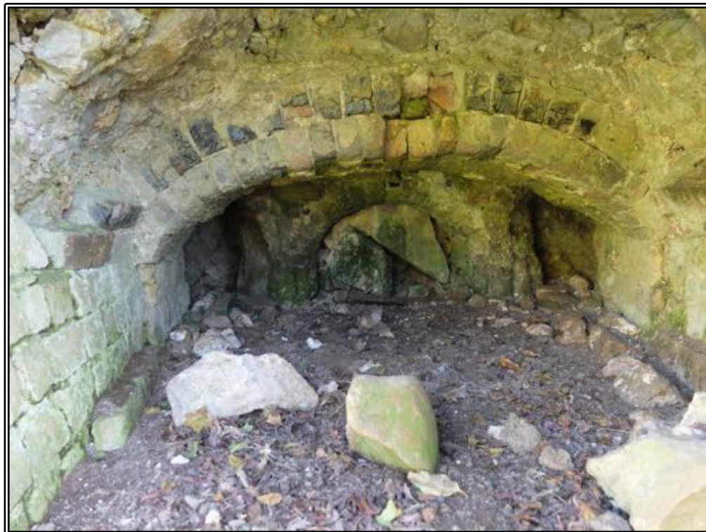
Figure 217 The firebox, showing the brick firebox arch and the three stoke holes.
