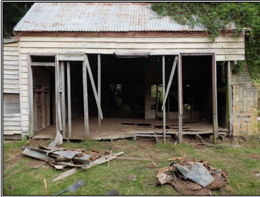
Figure 205 The front wall of the original section of Stewart's house, after the interior was cleared out. Despite the missing framing and cladding the front of the house is still standing reasonably square and level.
