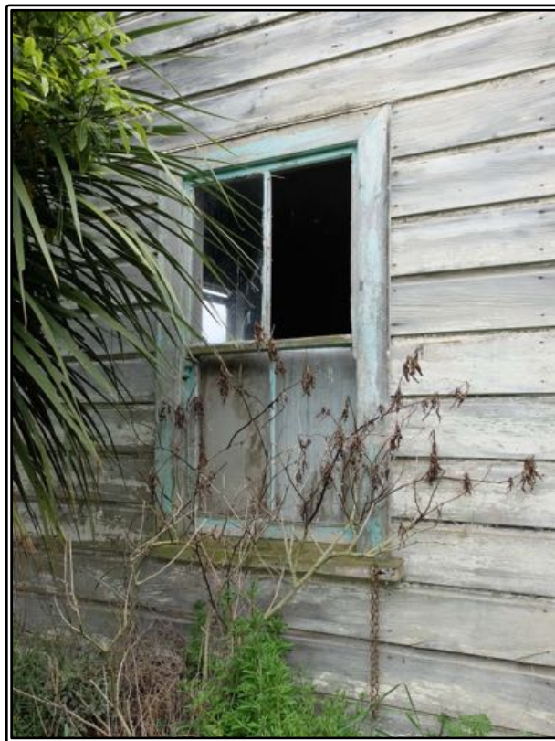
Figure 198 The original sash window in place in the eastern bay return of Roger's house.
