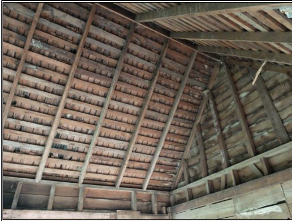
Figure 207 Looking up into the roof structure of the original part of Stewart's house. The timber shingles are all in place beneath the later corrugated iron.
