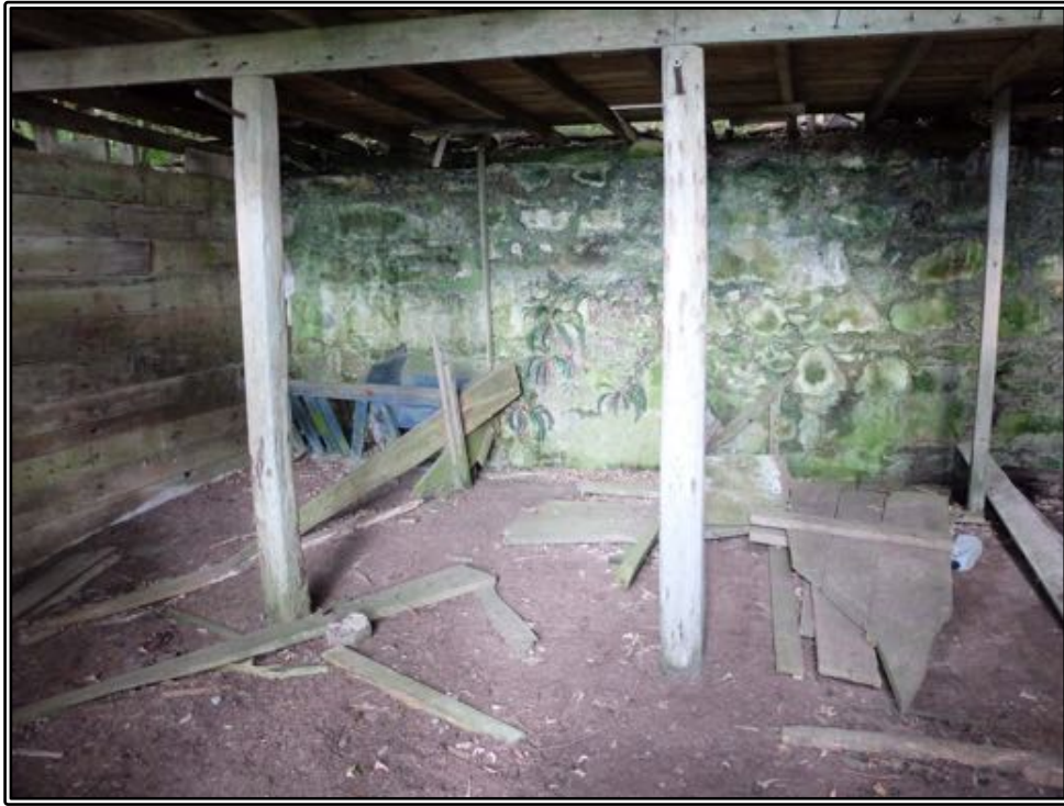
Figure 224 The stables section of Riddell's farm building, with the stone wall to the rear.
