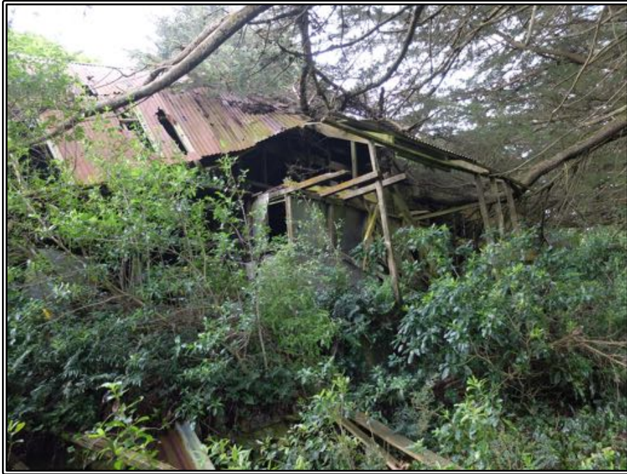
Figure 171 The front (east) of the building, showing the extension on the side where the Post Office was probably located.
