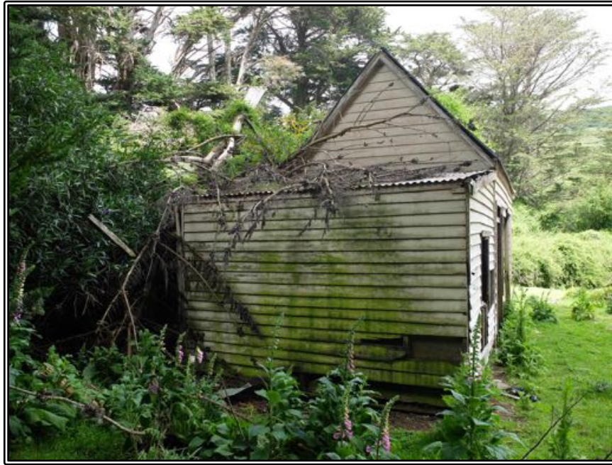
Figure 203 End view of the eastern end of Stewart's house, showing the later addition and the mass of fallen tree branches on the rear part of the structure.
