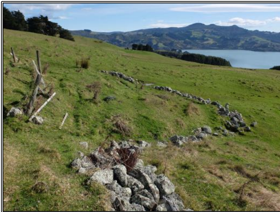
Figure 10 The section of wall I44/410 that has been displaced by slumping. Comparison with the image above taken in 1986 suggests that the ground may still be slowly moving.
