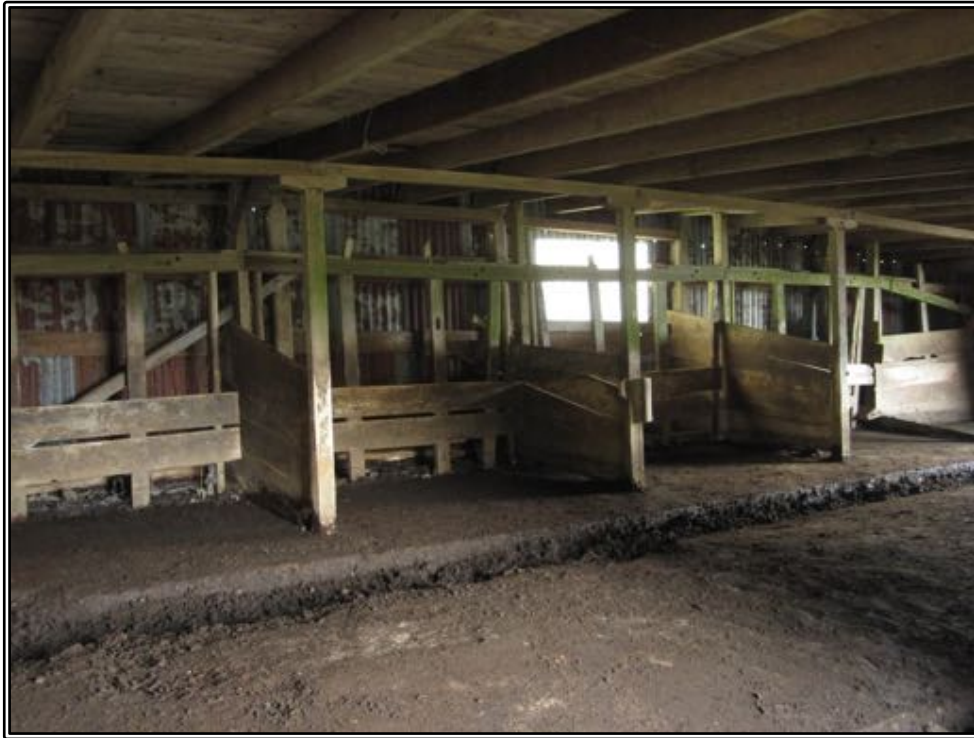
Figure 164 The original stalls in Larnach's byre exposed after the removal of the sheep pens in August 2017.
