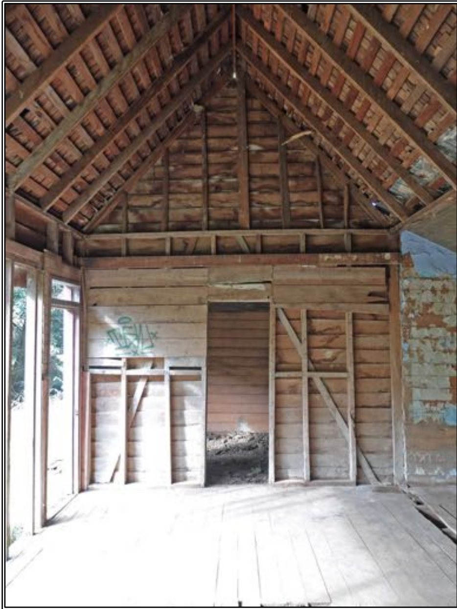
Figure 210 Looking towards the eastern end of the interior of Stewart's house after it was cleared out. A few scrim boards are still in place, but the wall framing is clear to see. The original pit-sawn weatherboards on this wall have been protected by the later extension built on the end of the cottage.
