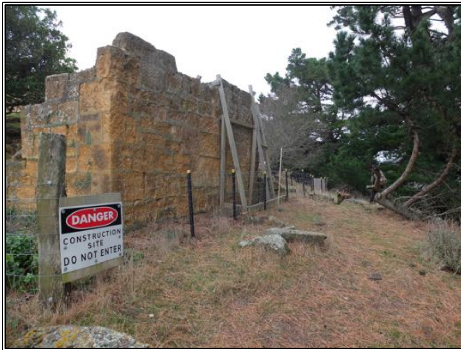
Figure 221 The end wall of Allan's house ruin in 2020 with timber props and safety fence in place.
