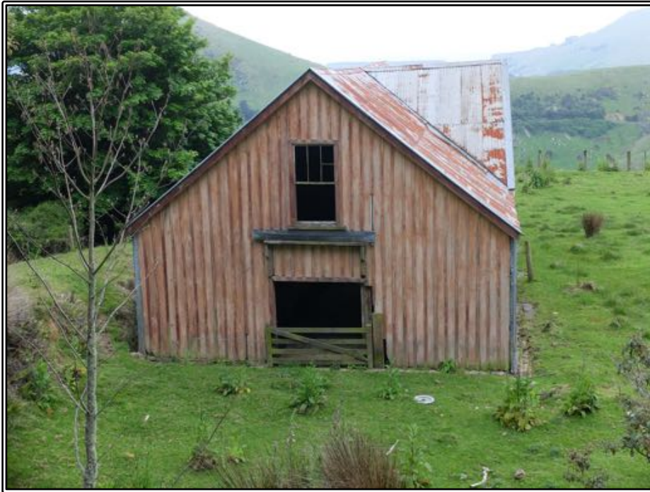
Figure 156 The western wall of Larnach's byre. The board and batten cladding is original, and all four walls were once clad this way. Note the window with the remains of a 6-light sash still in place.
