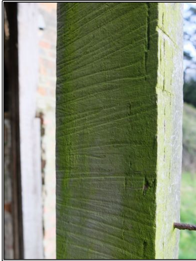
Figure 211 One of the framing studs of Stewart's house, showing distinctive pit-sawing marks.
