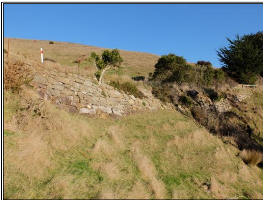
Figure 155 Stone revetment below Highcliff Road (I44/1014).
