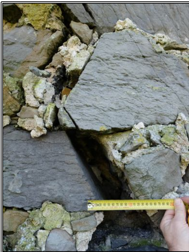
Figure 214 Close-up of one of the cracks in the charging bowl.
