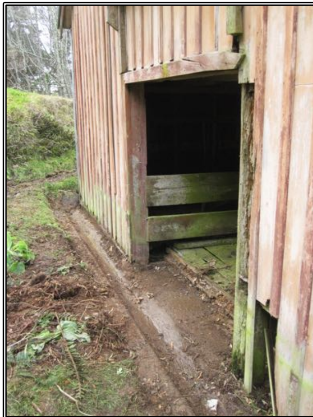
Figure 161 The external rainwater drain along the western wall of Larnach's byre after it was cleared out.
