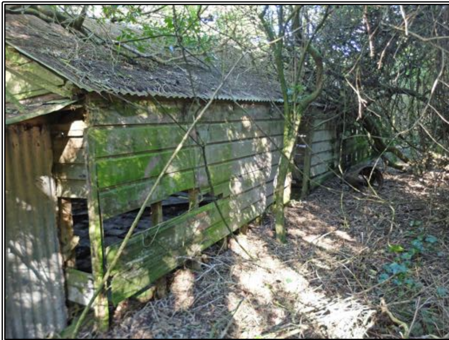
Figure 172 The rear wall of Riddell's farm building. This ground level is supported by a stone revetment, with the door in this wall opening into the upper floor of the building.
