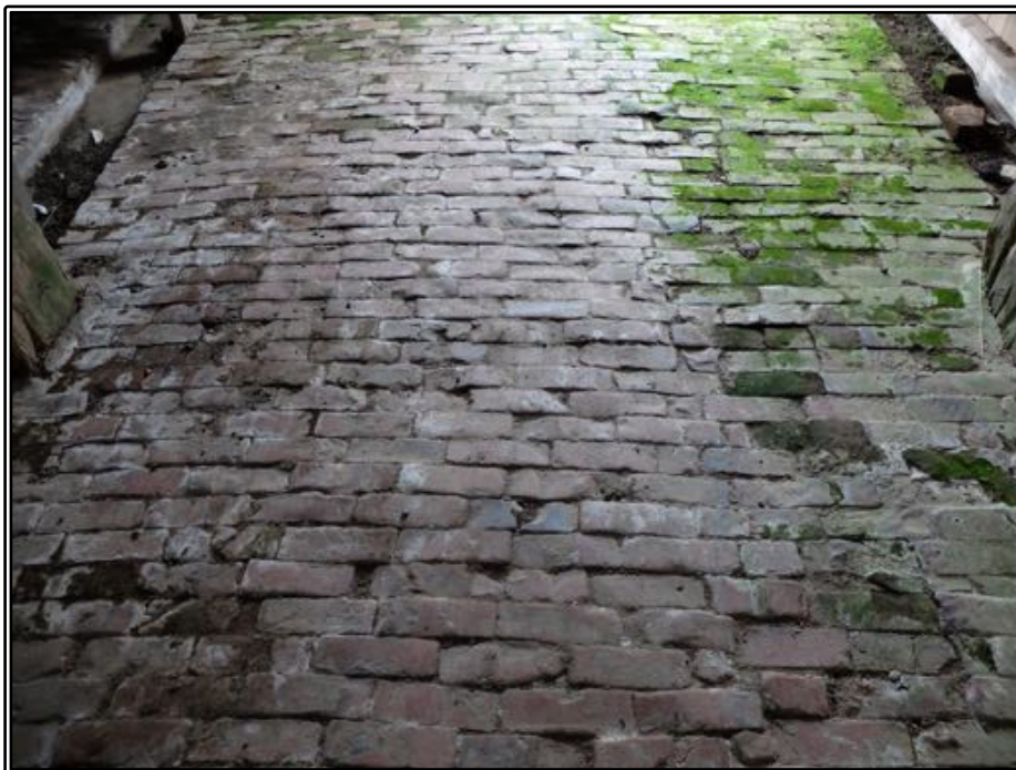
Figure 191 The central aisle of the brick floor, with a gentle hump to ensure drainage into the drains running along either side.
