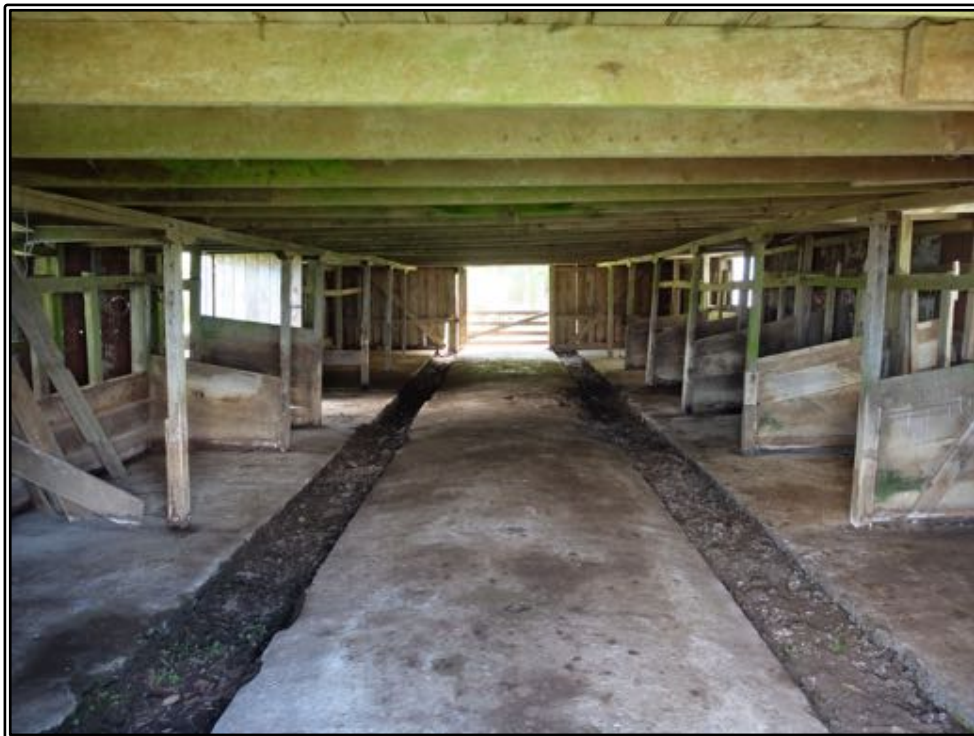
Figure 163 The interior of Larnach's byre after the sheep pens were removed in 2017.
