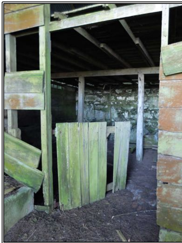
Figure 170 The stable door in the front (east) wall in 2017. Most of the vertical slats have now (2020) fallen off.
