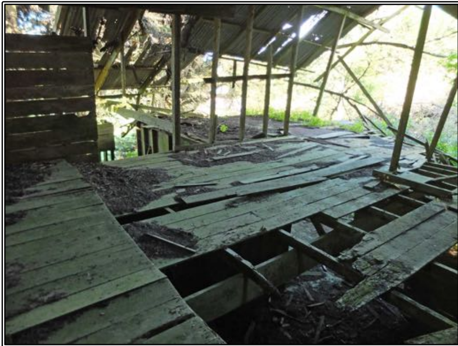
Figure 182 The upper storey in the southern surviving portion of Riddell's farm building.
