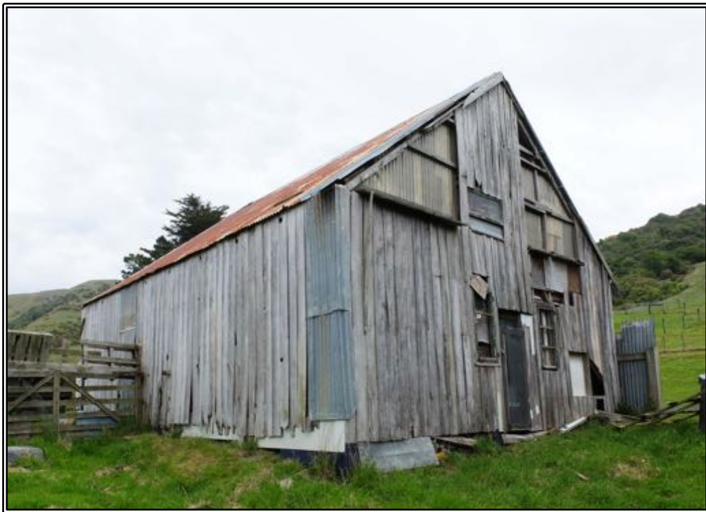
Figure 185 The east and north walls of Roger's byre. The original vertical board and batten cladding remains largely intact on these two walls. The cladding in the gable was probably cut away and replaced with transparent plastic sheeting when the byre was used as a chicken shed.
