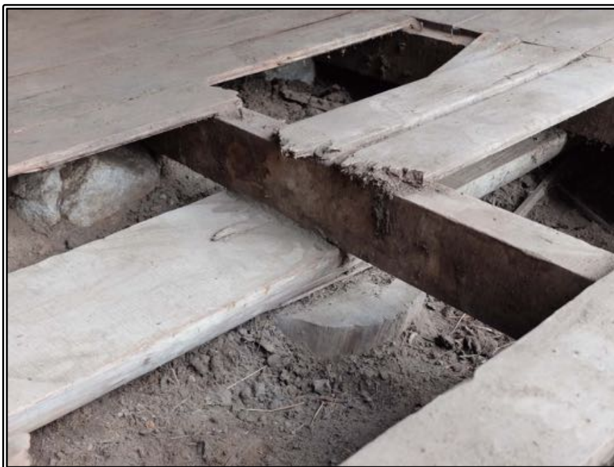
Figure 206 The sub-floor structure of Stewart's house where it has been exposed by broken floorboards. A full-round pile supports a half-round bearer, which in turns carries the floor joists and floorboards. All timbers are pit-sawn.
