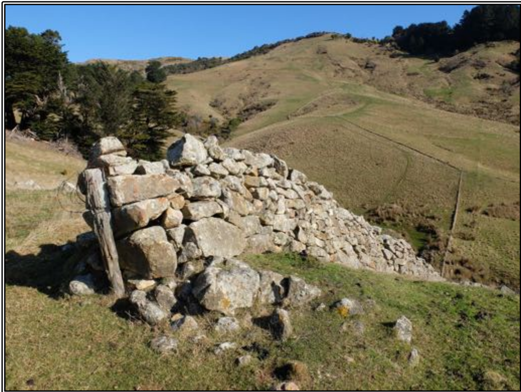
Figure 80 Gate end in stone wall I44/102 (Higham wall 4). It is the same gate end shown in the previous image, and it can be seen how the wall is leaning slowly to the left (south).
