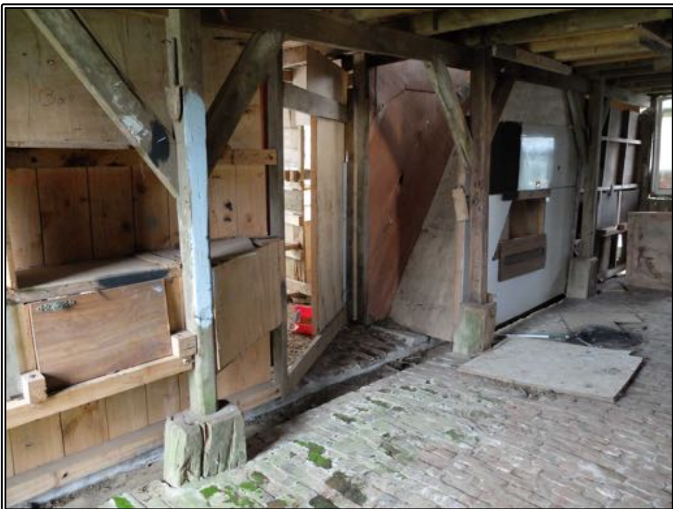
Figure 189 Inside the byre, showing details of the internal structure on the west side of the building, with the posts and braces intact, but with a mess of infill alterations in the stalls area.
