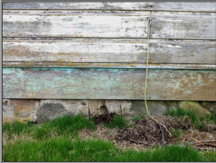
Figure 197 Detail of the base of the east side of the house, showing the hardwood piles and bluestone used in the foundations.
