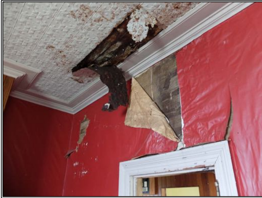
Figure 201 Inside the front eastern room of Roger's house, showing the effect of the leaking roof. The ceiling was pressed thin iron sheets over timber.
